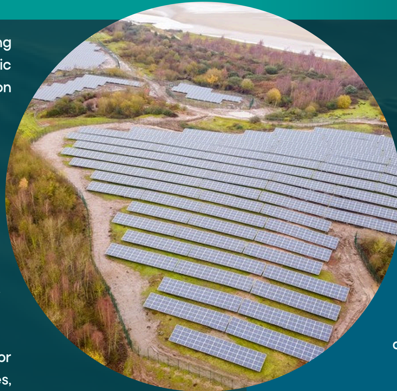
Figure 05: Crumps Yard, Connah's Quay Image: © SMA Solar Technology UK Ltd (Flintshire Solar Farm)
